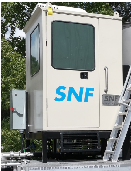
Control Room Cabin
