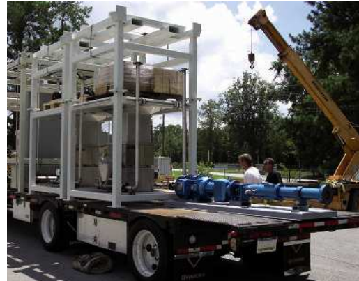
fig3 : skid mounted make up equipment
